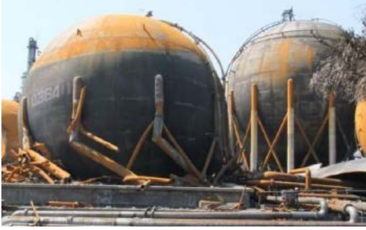
Fig. 1a. Earthquake consequences on a petrochemical plant (Japan, 11/03/ 2011)
